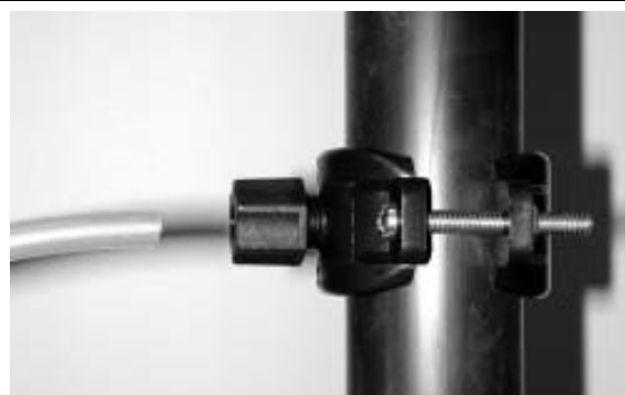
Drain Saddle (installed)
